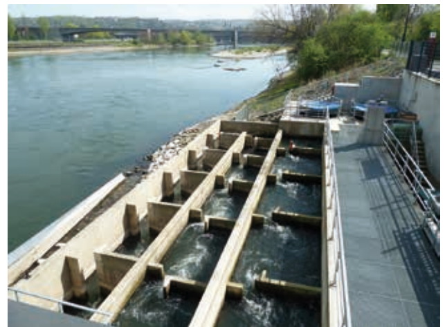
Fish ladder on the Koblenz barrage weir on the Moselle Source: Stephan Naumann
